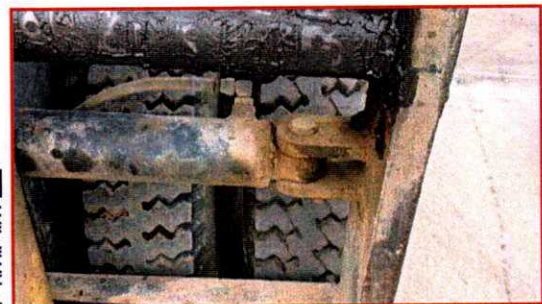
6- Control unit hydraulic Hose the condition satisfactory at the time of inspection
